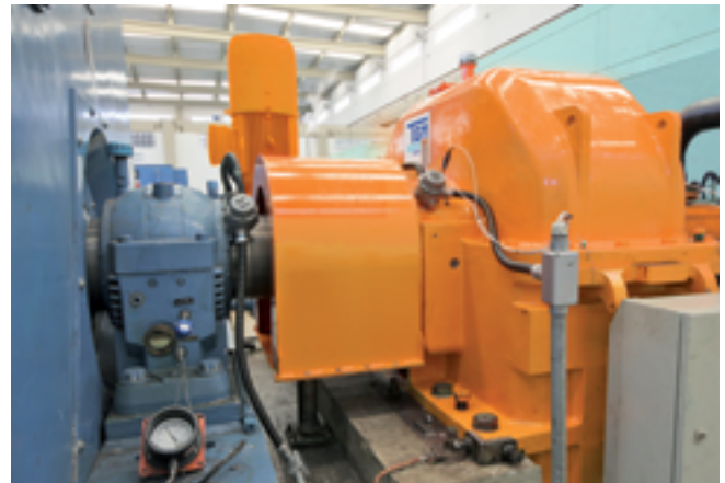
CMAA Vale do Tijuco - Uberaba, MG - Brazil / Turbogenerator - 49 MW SuperTurbo - ST 630
