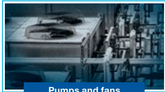
Pumps and fans
