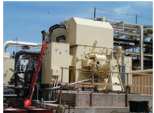
Dresser-Rand – Arizona Public Service – USA 52500 kVA, 2 Poles, 3PH / 60 Hz / 13.8 kV
