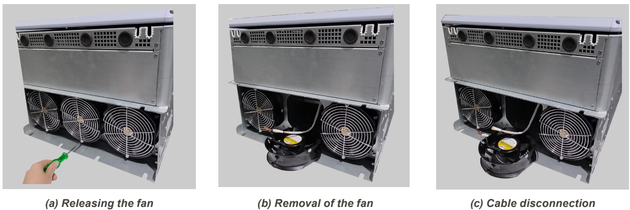
Figure 6.3: (a) to (c) Removing the heatsink fan (Frames E, F, G and H)
