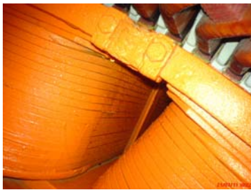
Figure 26: Humidity on the windings
