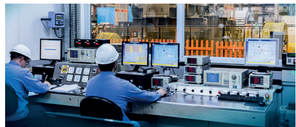
20 MVA test lab monitoring room
