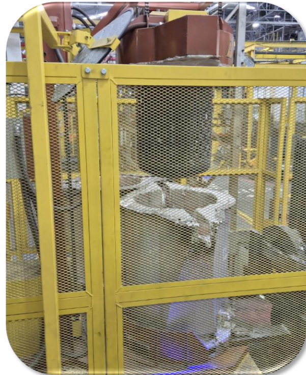
Electric ladle heater at the Aluminum Injection area
