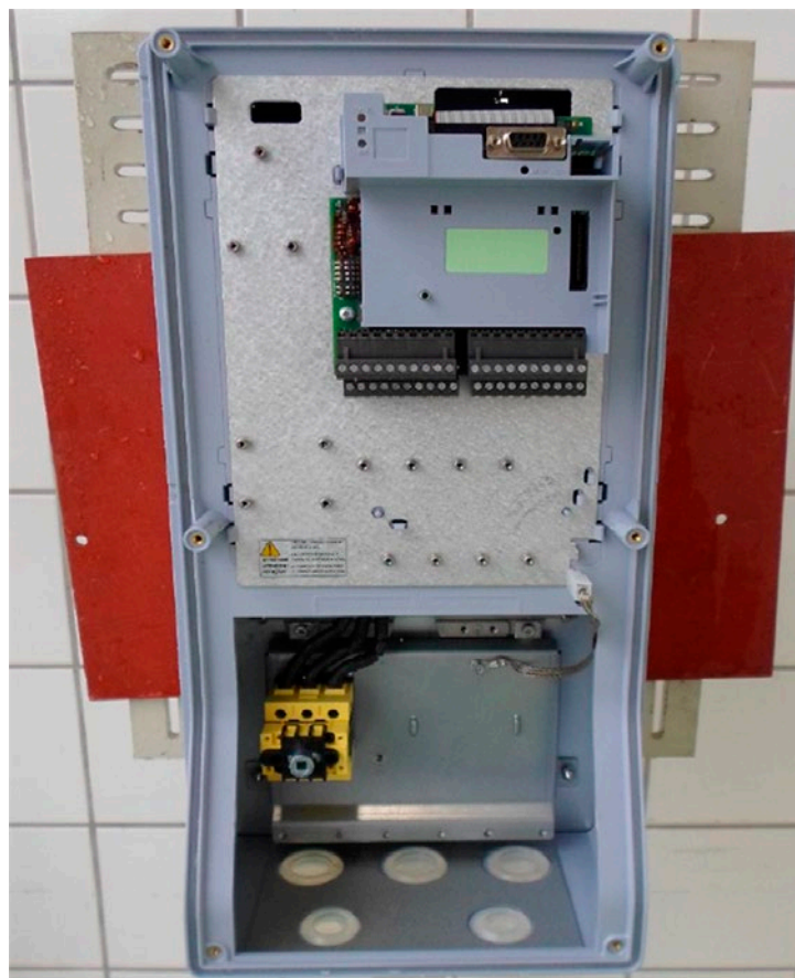
Sample 01 internal side after water ingress test; Control board and input
