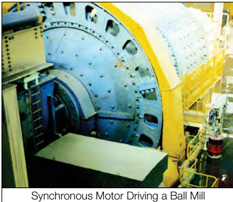
Synchronous Motor Driving a Ball Mill
