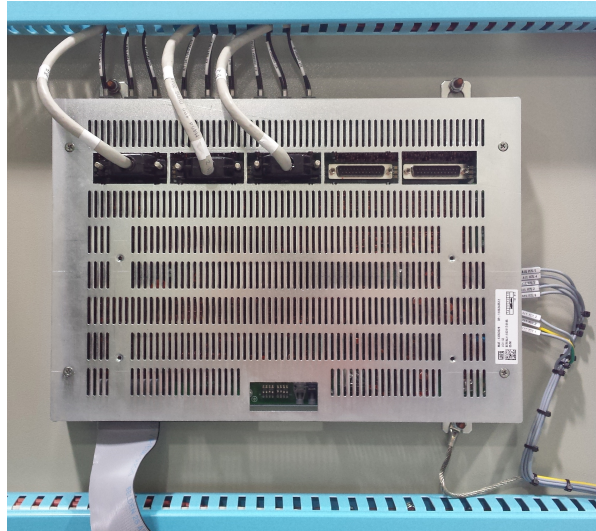
Figure 3.37: ICUP shield fastened to the panel
