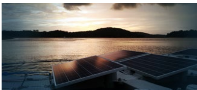
Flutuante - 1 MWp - CHESF
