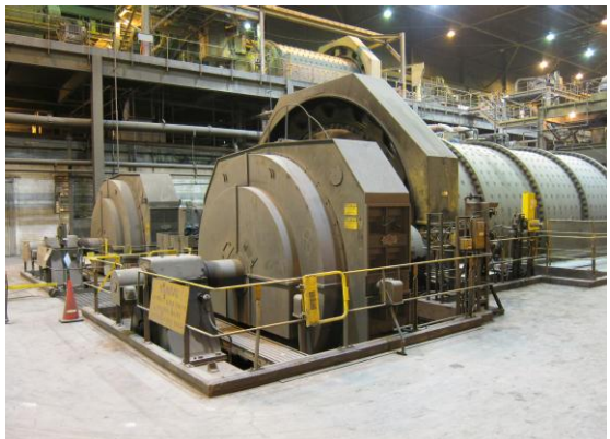
United Taconite LLC – Minnesota USA Load sharing Ball Mill 3000HP, 44 Poles, 3PH / 60 Hz / 4.0 kV
