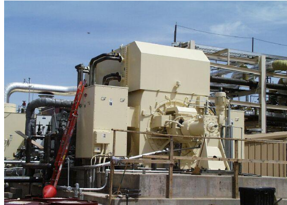
Dresser-Rand – Arizona Public Service – USA 52.500 kVA, 2 Poles, 3PH / 60 Hz / 13.8 kV
