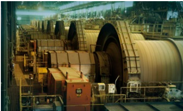
Codelco Teniente - Chile Single pinion ball mills - LSS Motors (Retrofit)
