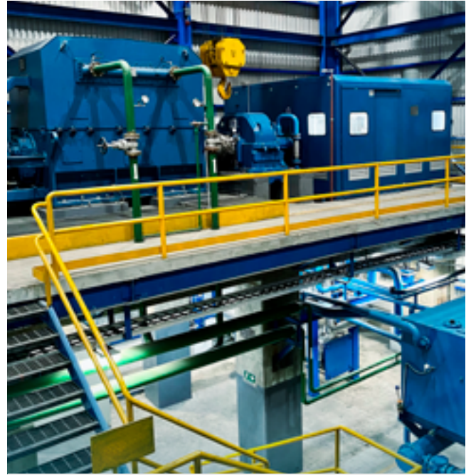
Higher level installation with civil base, downward radial exhaust and 4-pole generator.
