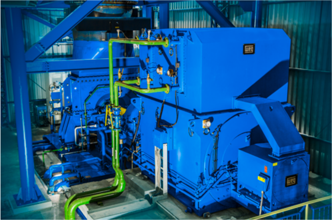
Ground level installation with metallic base, radial exhaust upwards and 2-pole generator.
