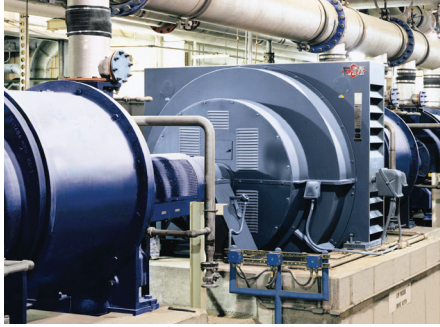
Vacuum pump drive
