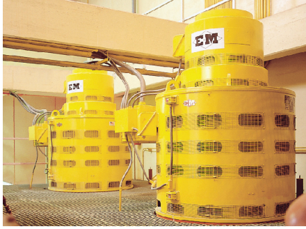
Variable speed municipal pump drive.
