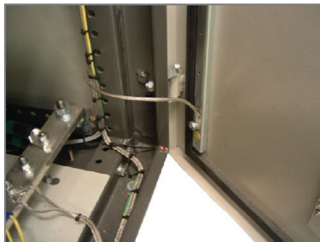
Figure 3.39: Grounding of the panel door
