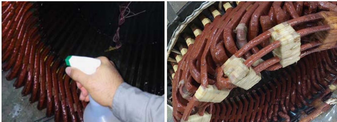
Figure 12: Sample of high voltage stator - Contaminated (Source: WEG)
