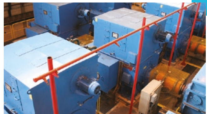
Synchronous motors SDL800, 3,000 kW, 3,100 V Application: rolling mills (iron and steel)
