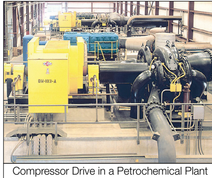
Compressor Drive in a Petrochemical Plant
