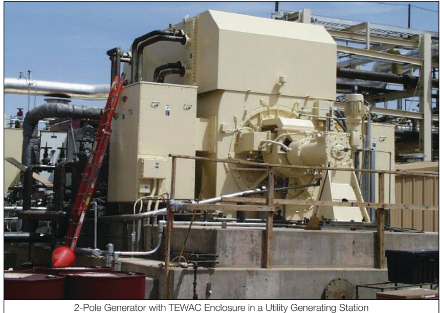
2-Pole Generator with TEWAC Enclosure in a Utility Generating Station
