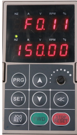
Figure - HMI of Inverter
