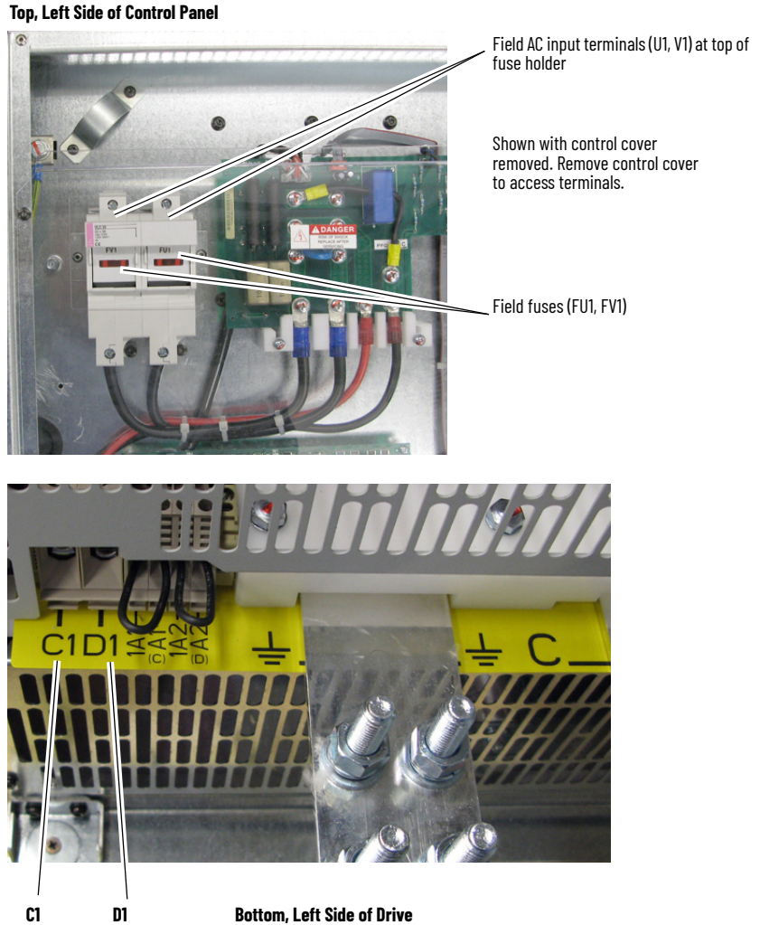
Figure 14 - Field Terminal Block and Field Fuse Locations
