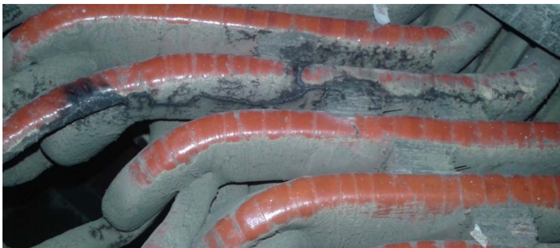
Figure 2: Tracking on the contaminated insulation surface
